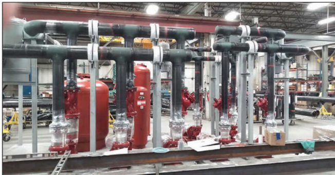
Harris' work on the 668,000-square-foot Heywood Bus Garage project included prefabricating a massive pump skid. The 21-foot by 10-foot skid weighing roughly 15,000 pounds houses the base-mounted pumps, expansion tanks, air separators and pot feeders for the chilled water, ground source water and heating water systems running the building. Photo: Harris.
